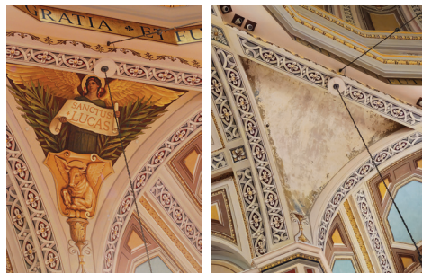
This large image of St. Luke fell from the ceiling about four years ago. The Cathedral has been collecting funds through a second collection on the first Sunday of the month to support the restoration of this piece and other sacred artwork.
