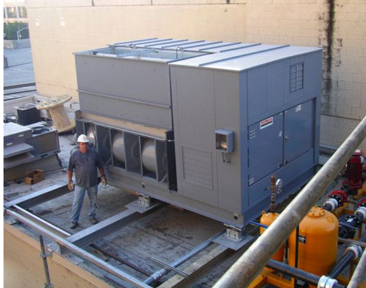
THIS 18,000-POUND CHILLER WAS RECENTLY PLACED ON THE ROOF OF THE MANOGUE BUILDING. CHILLED WATER FROM THIS UNIT WILL PRODUCE THE COLD AIR THAT WILL COOL THE CATHEDRAL.
